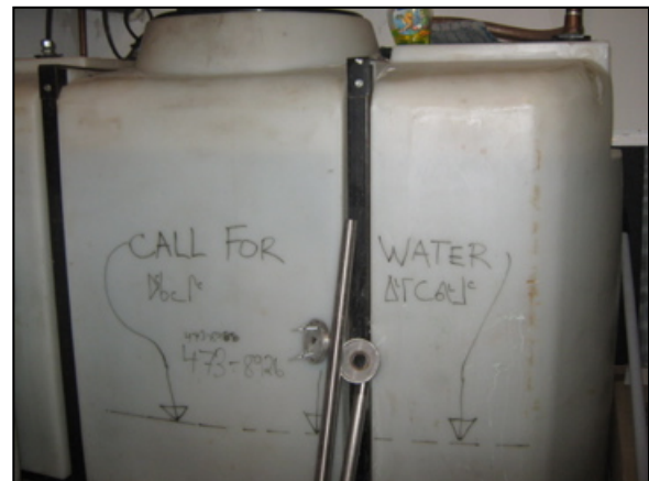
Fig. 1. Household water tank in Nunavut.
